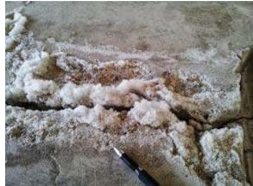
Efflorescence, salts being "purged" out of the slab by the action of the CMW
